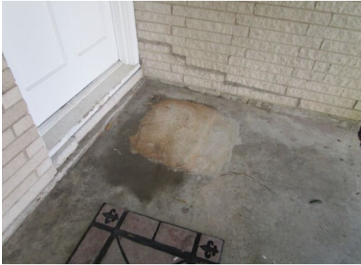
Signs of previous foundation repairs
