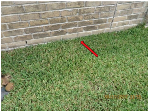
4in clearance between soil and brick is missing
