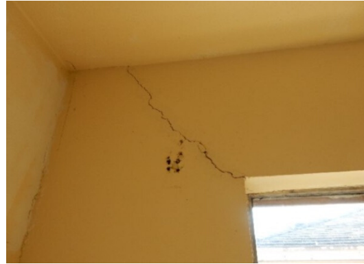
Typically signs of foundation issues
